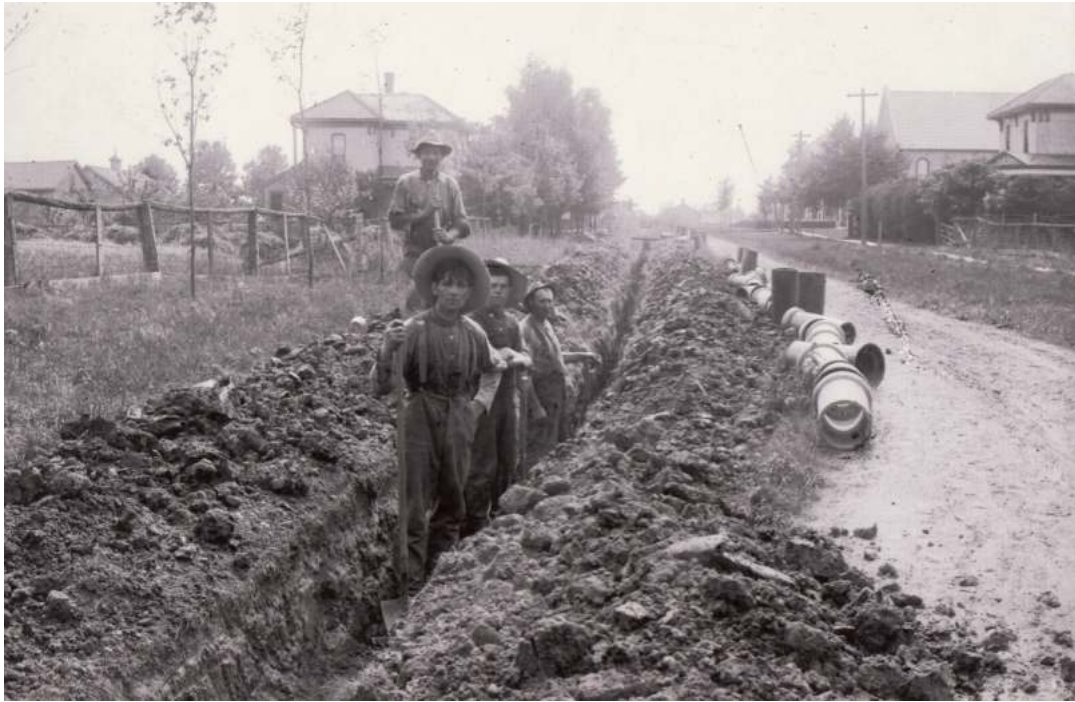
Construction on Oxford Street (LSC) ... 22 Oxford is on the right Sidewalks were laid on the south side of Oxford Street in 1913. It's not known if this picture relates to that work or is from an earlier time.
